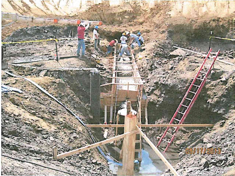
Photo 1.: New Secondary Clarifier No. 3's center lower hub 20" ductile iron RAS, southwest alignment, being concrete encased between bulkhead forms (looking southwest)
