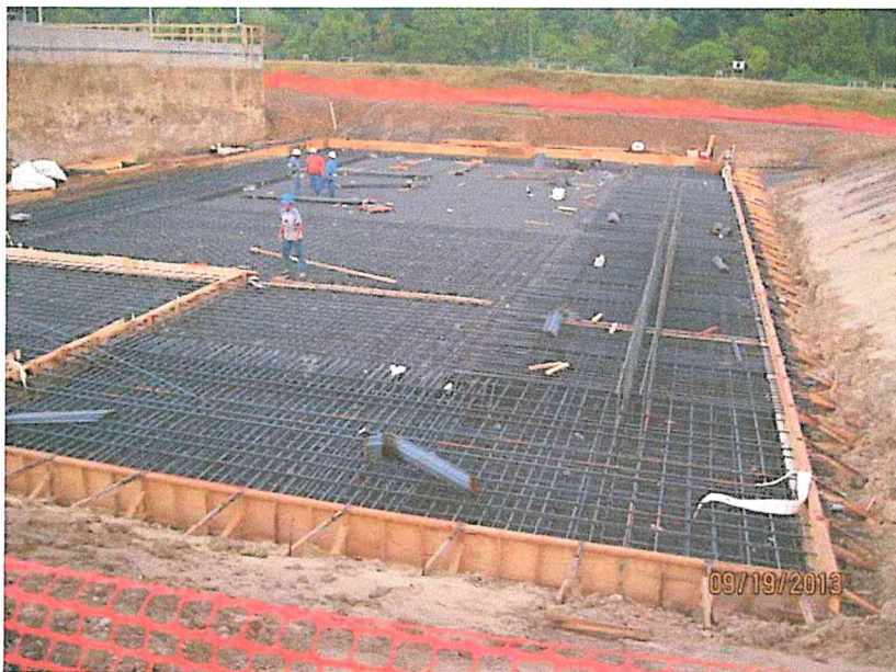
Photo 3.: New Aeration Basin No. 3's foundation slab receiving lower & upper mats reinforcement steel also vertical wall hook dowels. Along the south slab edge (formed) is the reinforced 22" thick x 20" length knock-out slab extension (future AB connection), (looking east)
