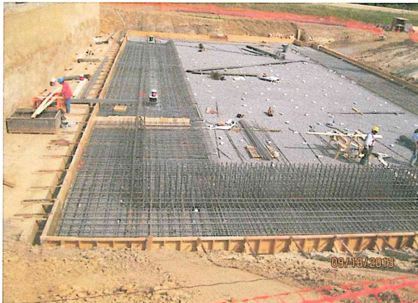
Photo 2.: New Aeration Basin No. 3's interior foundation and perimeter thickened spread footer slabs (8 ea.), above compacted #57 stone receiving lower & upper transverse & longitudinal rebars between bulkheads including waterstops (looking east)
