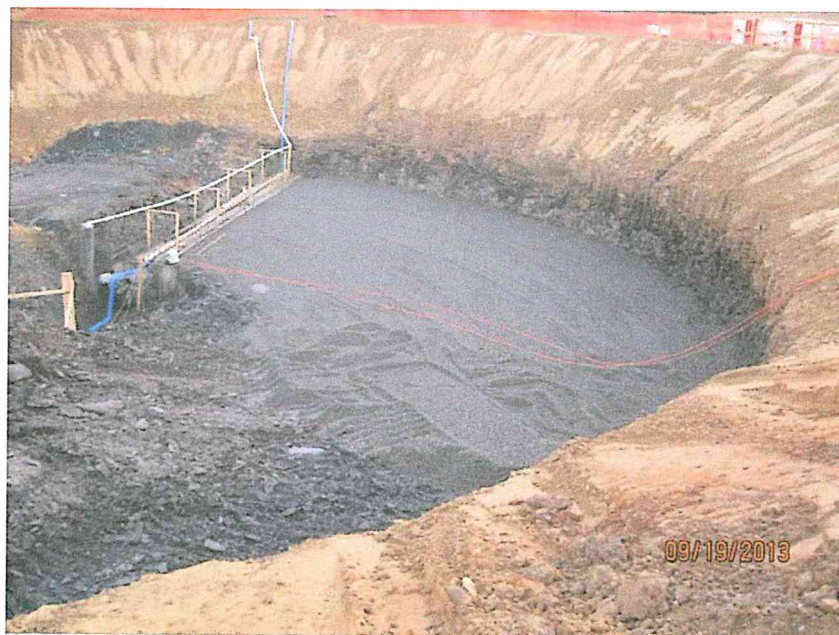
Photo 4.: New Secondary Clarifier No. 3's foundation slab's rough grade excavated shale rock bottom. Below 6" concrete seal slab compacted #57 stone base placed to adjust slope at 12:1. Concrete encased 20" DI RAS from center hub in background (looking south)
